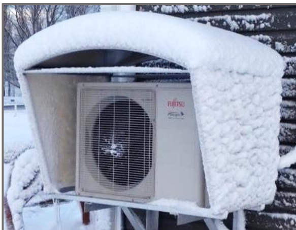
Figure 39: Fujitsu heat pump in the snow. 86
