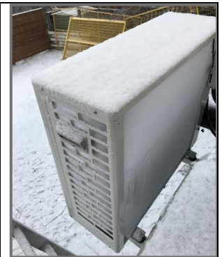
Figure 41: A Sanden CO2 heat pump water heater compressor working outside in 5°F (-15°C) weather. 89
