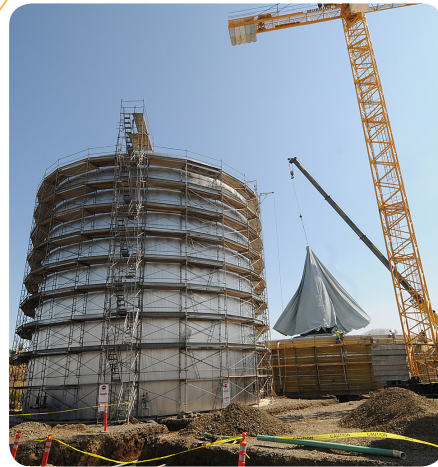
The continuously stirred tank reactor, CSTR, where heated waste digests in an oxygen-free environment, takes shape on left. Smaller crane on right hoists inflatable top for the biogas storage tank.
